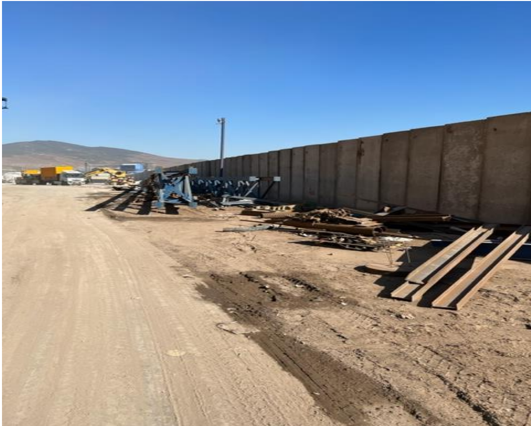
Photo-8: Construction Waste and Dust Accumulation on the Ground
