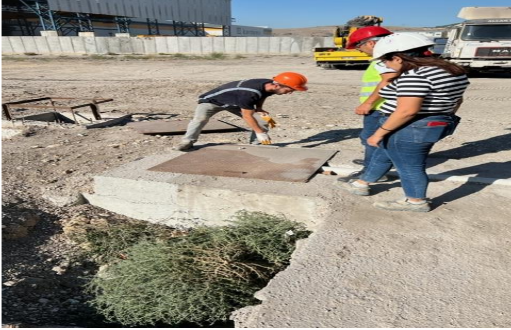
Photo-11: Drainage Well in the Waste Storage Area
