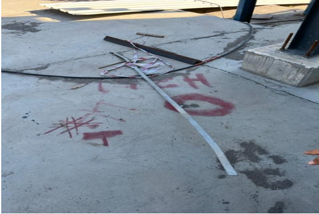
Photo-7: Unproper Material Storage
